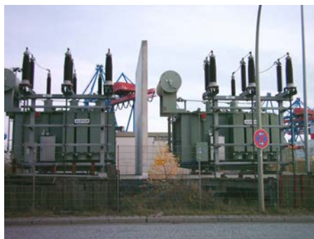
Figure 20.22 Power is distributed over large distances at high voltage to reduce power loss in the transmission lines. The voltages generated at the power plant are stepped up by passive devices called transformers (see Transformers ) to 330,000 volts (or more in some places worldwide). At the point of use, the transformers reduce the voltage transmitted for safe residential and commercial use. (Credit: GeorgHH, Wikimedia Commons)
